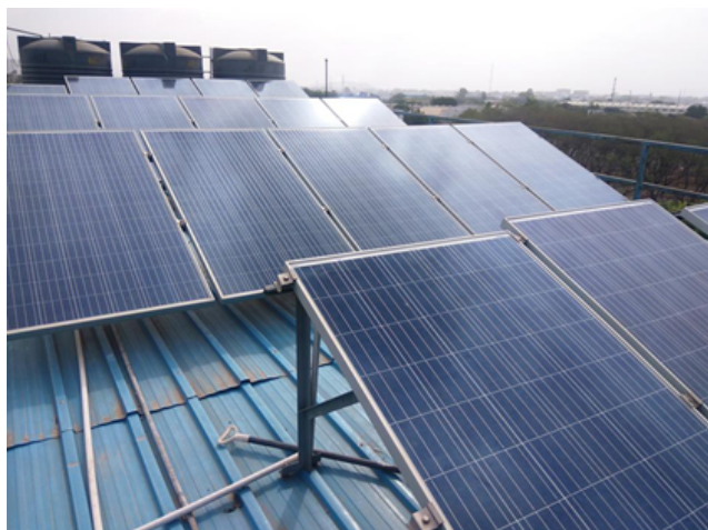
Figure 1: A photograph of rooftop mounted 6 kW solar PV plant.
