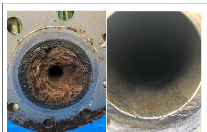
Figure 3: Pipeline congested with paraffin (left) and then after remedial chemical treatment (right).
