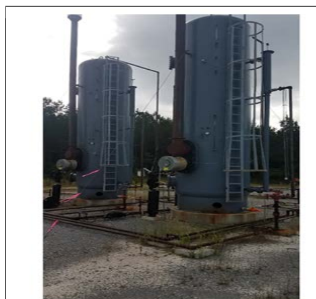
Figure 4: Example of a goodrich heater treater.
