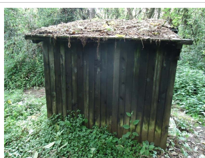
Figure 4: A picture showing outdated type of toilet (temporary toilet).
