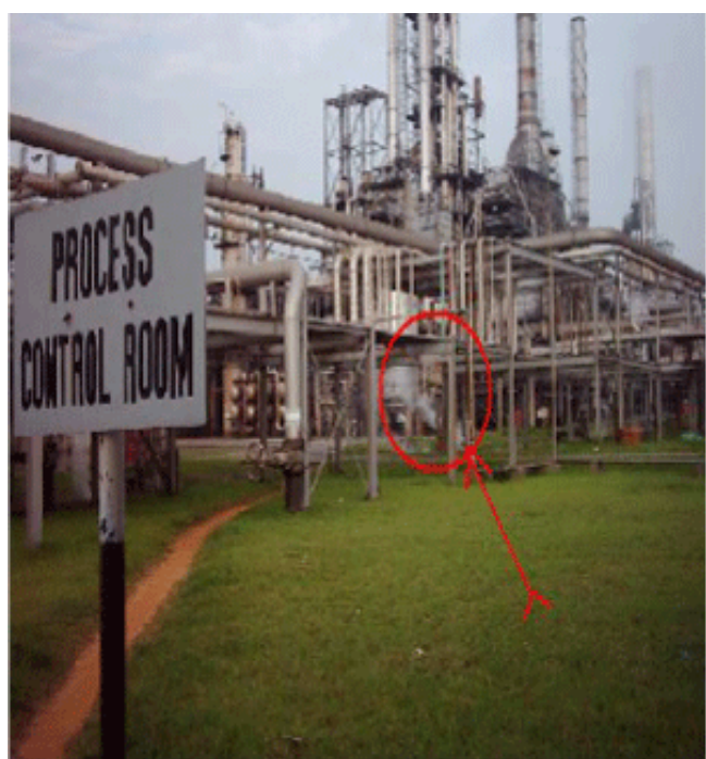
Figure 2: PHRC PLANT UNIT: Notice the highly pressured misty discharges from one of the defective valves – A common sight in many processing units of PHRC Plant.
