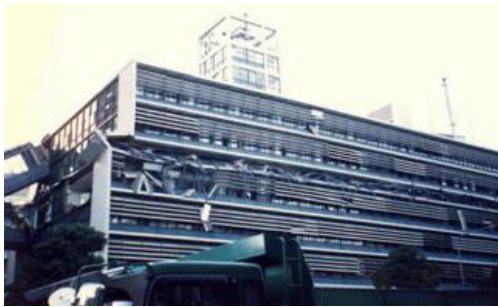
Figure 2: Mid-story failure of Kobe city hall during the 1995 Kobe earthquake.
