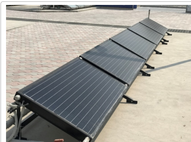
Figure 3: Photographic view of solar PV/T hybrid collector system set connected in series within a closed hydronic circuit at the Techno Hub facility, Gulf organization for research and development, Qatar (latitude 25.3548° N).
