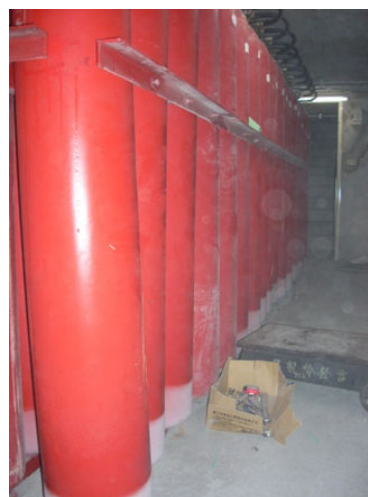
Figure 1: Liquid carbon dioxide steel cylinders in basement.
