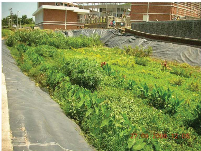
300,000 lit/day Composite Sewage Reed Bed System Symbiosis Knowledge Village, Lavale, Pune
