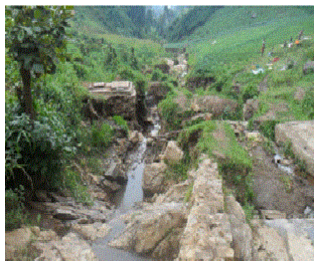
Figure 3: Destroyed gravity water source in Rutegyengyere.
