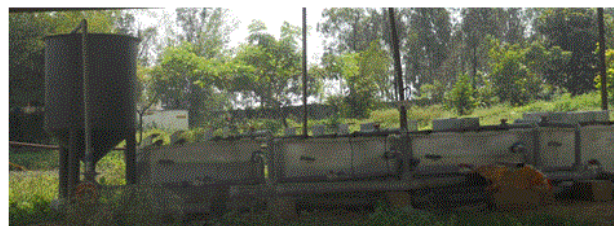
Figure 8: Reverse osmosis process carried out in landfill.
