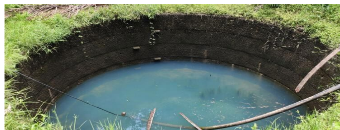
Figure 2: Poorly constructed irrigation wells.
