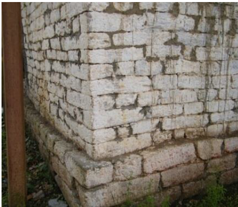
Figure 20: Shear cracks and bulging of wall in bending.
