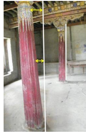
Figure 22: Bulging in columns.
