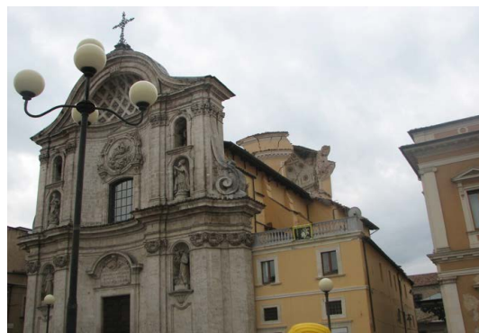
Figure 3: The Church of Santa Maria del Suffrajo in the town of Aquila, damaged after the seismic impact of the earthquake in 2009.
