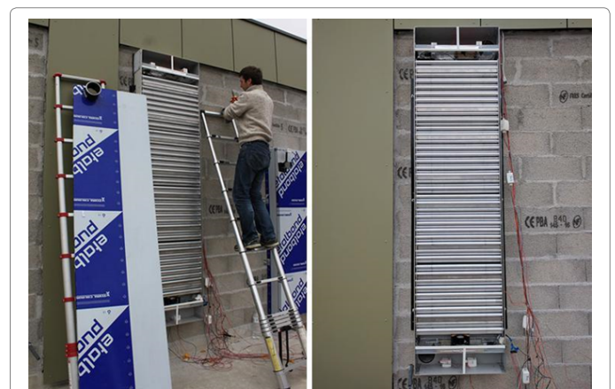
Figure 2: Installation of the LHTES on the BEF cell.
