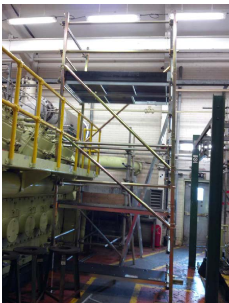
Figure 2: Tower 2: 2.4 × 1.4 × 4 m, 2 Standards offset on gantry of Compressor K40.
