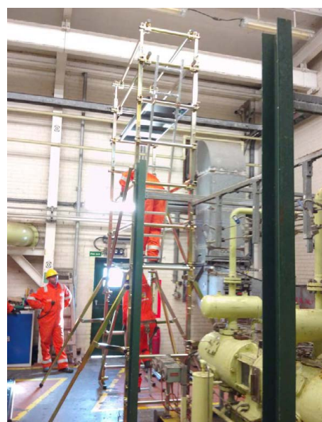
Figure 4: Tower 4: 1.8 × 0.8 × 4 m, Erected in clear area between K710 Skid and K10 compressor.
