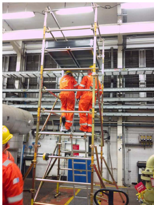
Figure 1: Tower 1: 1.8 \times 1.7 \times 4 m, Erected in clear area between K2710 Flash Gas Skid and K40 Compressor.
