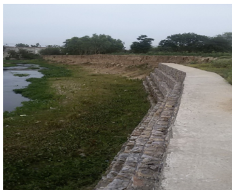
Figure 1: Stream bank erosion and retaining wall at Maneri.
